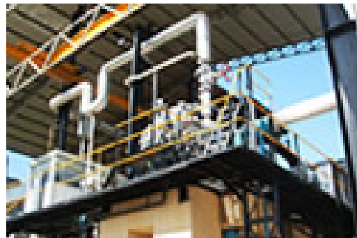
The Steam Turbine of the 1 MW Grid Connected Biomass Plant at Walapane, Sri Lanka
